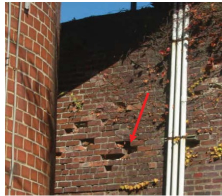
Photo 10- Deterioration and spalling of bricks in electrical vault wall due to water intrusion
