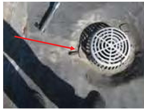
Photo 36- separation of roof membrane at roof drain penetration
