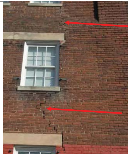
Photo 18- South-SE corner structural crack between 1 st and 2 nd floor & 2 nd to 3 rd floor
