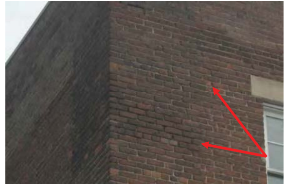
Photo 14 – South-SW 3 rd floor corner needs masonry tuck pointing
