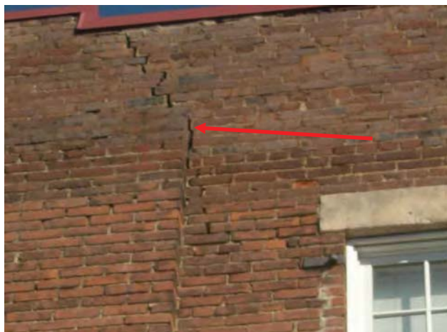
Photo 17- South-SE corner cracking continues 3 rd floor to roof parapet
