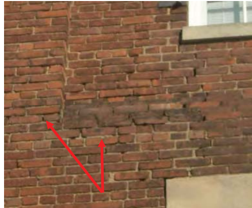
Photo 16- South elevation – Crack repair and tuck pointing needed.
