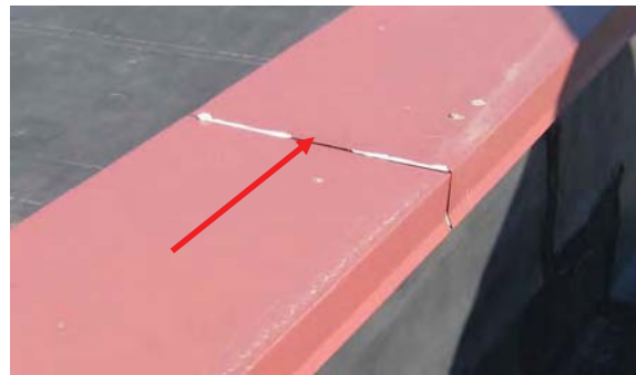
Photo 42- seams at parapet flashing need re-caulking
