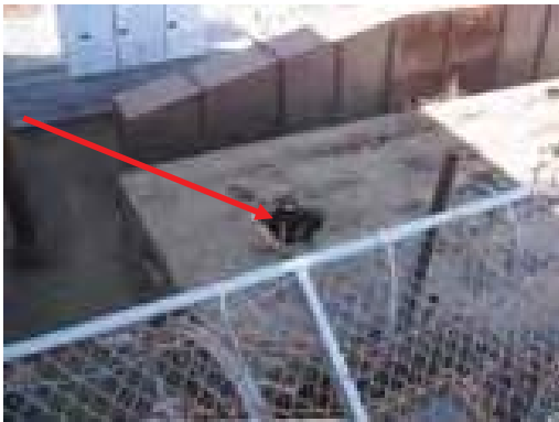
Photo 39- Hole in roof of east in of boiler room.
