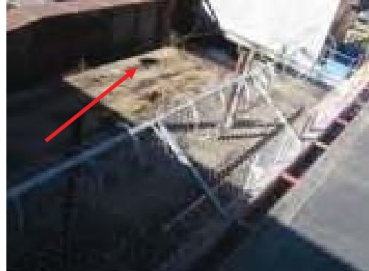
Photo 40- Hole in roof of west end of boiler room.
