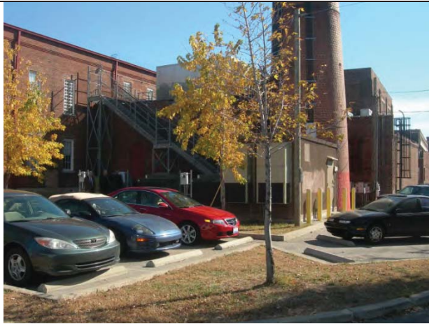
Photo 9 – Electrical transformers, electrical vault and smoke stack west elevation
