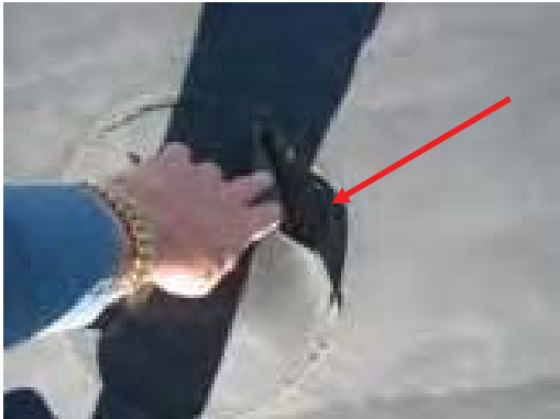
Photo 35- separation of roof membrane at penetration
