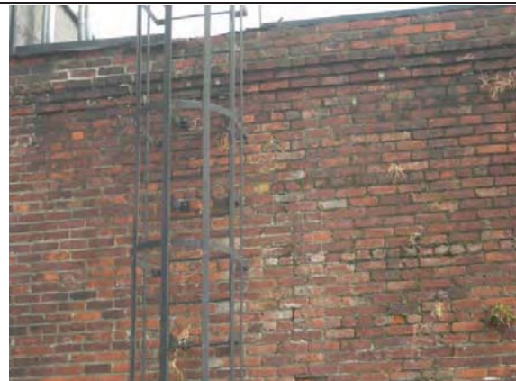
Photo 12- Old boiler room wall has multiple locations with plants growing on vertical face which means significant intrusion of water into mortar joints.
