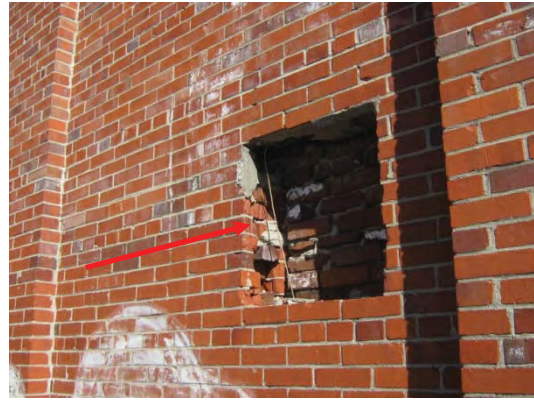
Photo 38 - Recesses in parapet walls allowing water intrusion into parapet wall.
